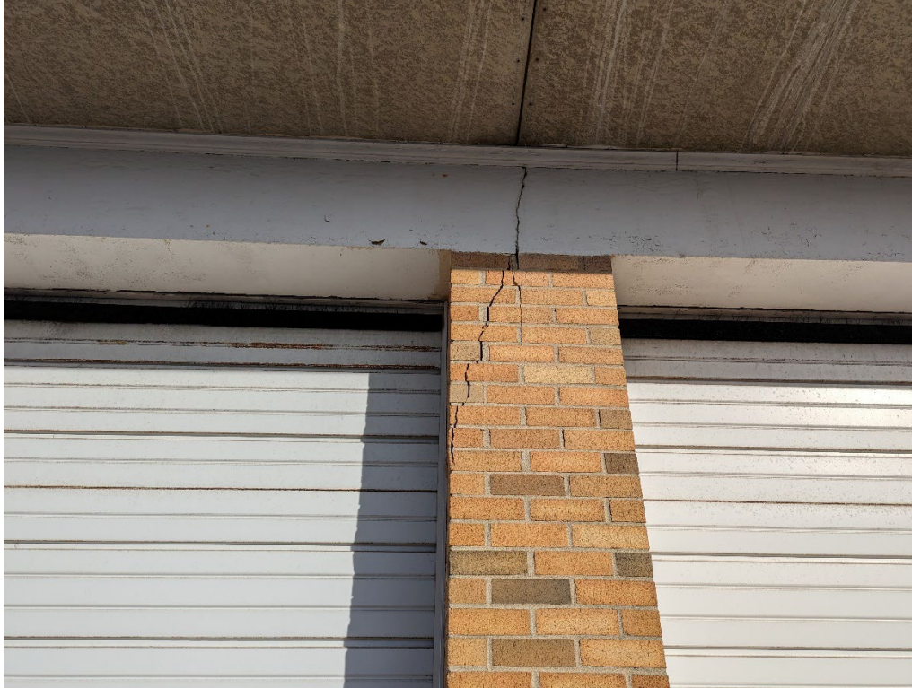
Image 16 - Cracking in the bus garage brick / masonry
