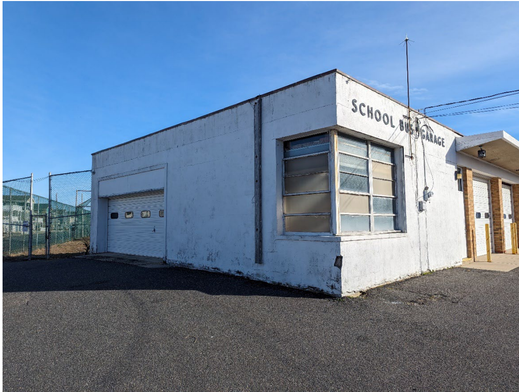
Image 18 - Bus garage and northern bay, some foundation and facade damage is evident
