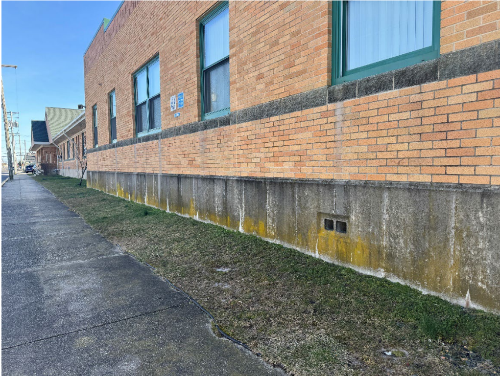
Image 2 - Flood vents and foundation wear along West 19th Street
