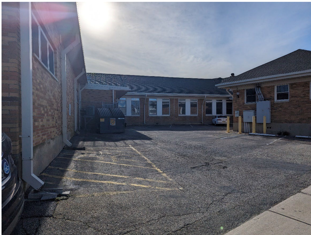
Image 3 - Small parking lot with un-enclosed dumpster, uncontrolled downspouts, and limited circulation
